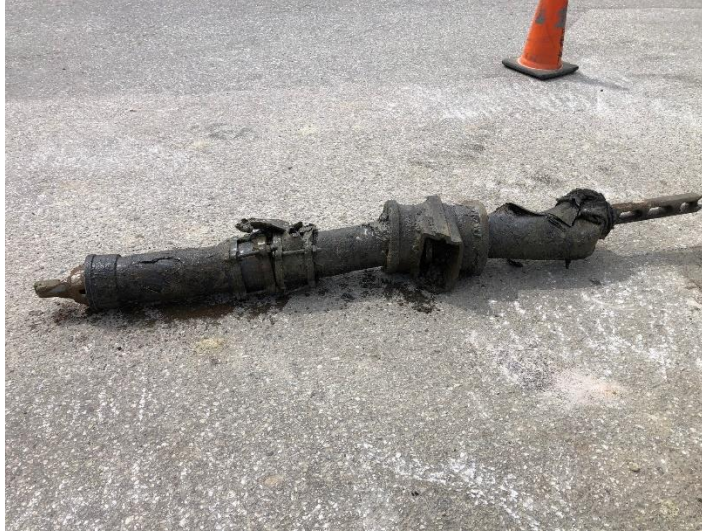
Figure 5 - An example of old infrastructure encountered that might have been shared by a long-time operations employee.
