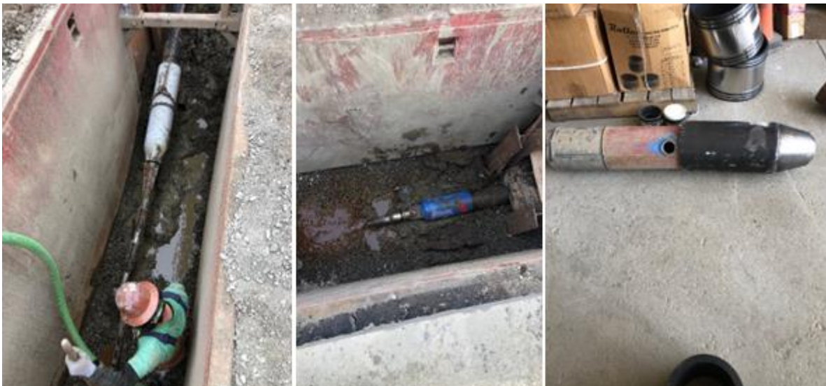
Figure 4 - The three bursting head options; the white head is a manufactured supplied head that was too large, the blue head is an HDD pulling head which was the same OD as the host pipe and too small, the black head was PW's design which worked.
